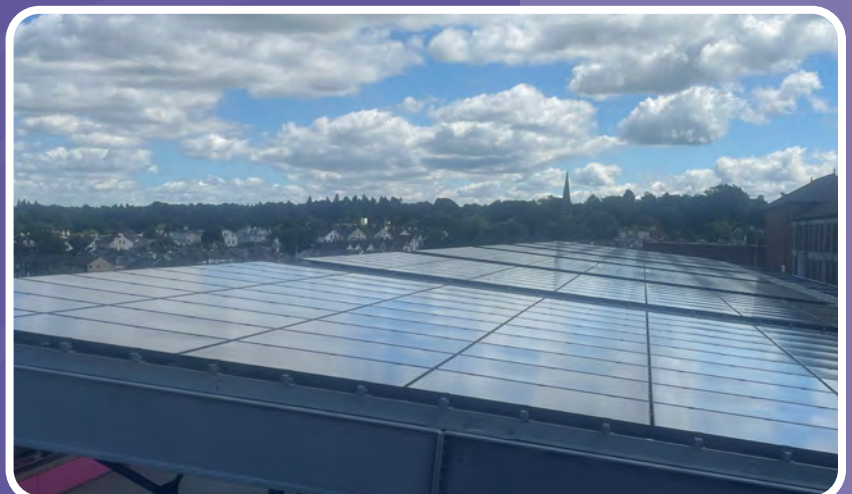
973 solar panels installed on RVP car park roof
